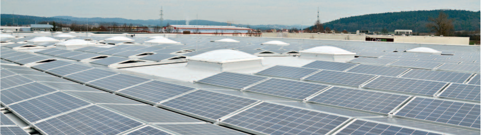
The panels on the roof of Aumüller Druck are at a flatter angle than usual, which means that they cast less of a shadow on each other.
