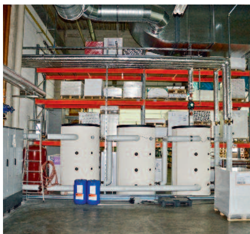
Inverter heat pumps have been installed to reduce current operating costs.
